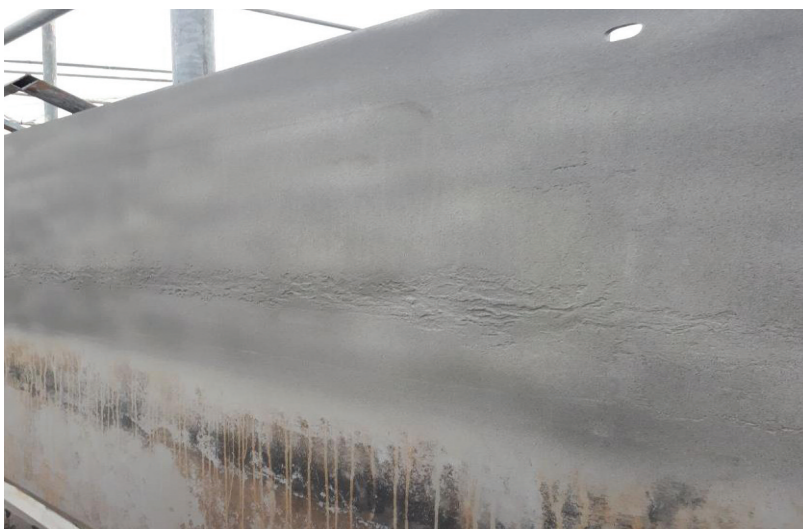
The reactor wall after blast cleaning showing the anaerobes damage
